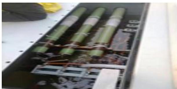
箱变熔断器损坏
